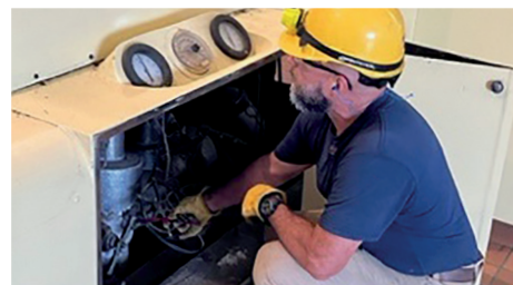
Above | Carlos Garcia, shift operator, Corn Belt Power Cooperative, adjusts sealing steam on Wisdom Unit 1 during August operations.
