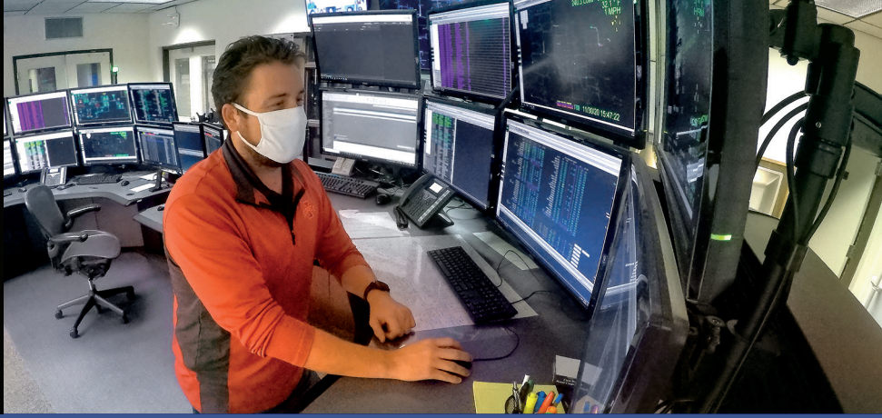
Above | Tom Hanrahan, system operator, monitors system interconnections in the control center late November.
