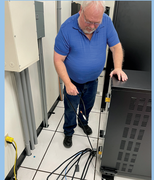
Above | Dennis Anderson, information technology administrator, Corn Belt Power connects the new UPS system.
