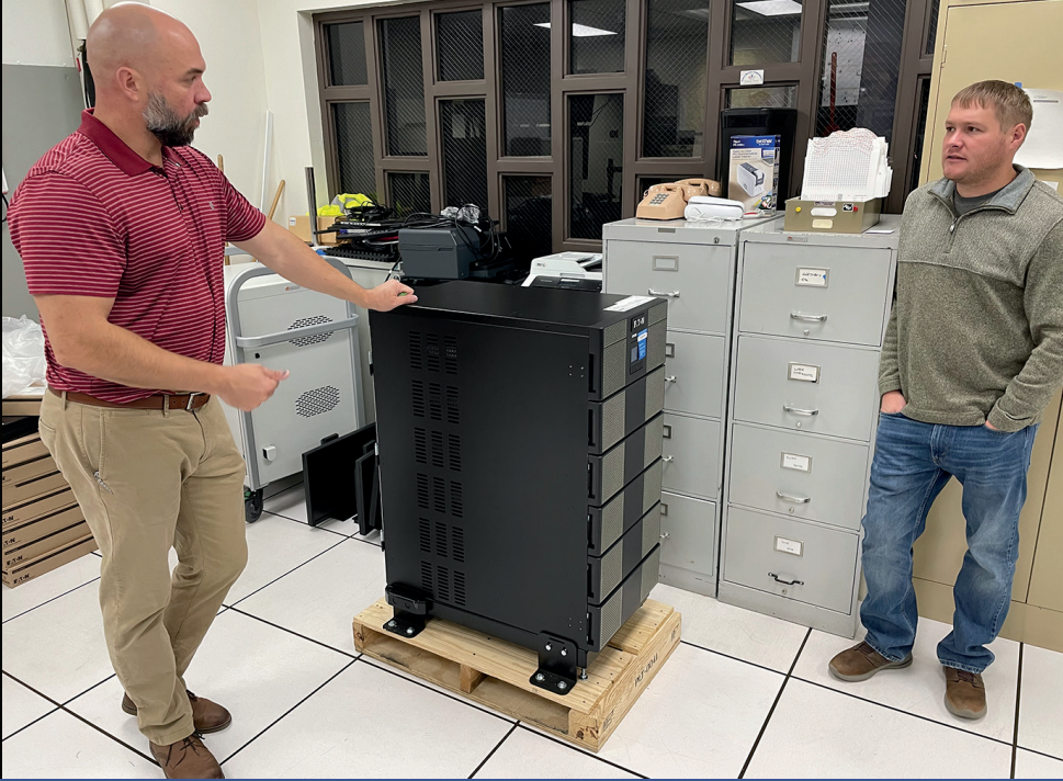
Above | Jon Myer, left, information technology administrator, Corn Belt Power, and Jon Behounek, chief system operator, Corn Belt Power, discuss the installation of the cooperative's new uninterruptible power supply (UPS). The UPS device will help ensure continuity of services in the case of a power outage at Corn Belt Power's corporate headquarters.
